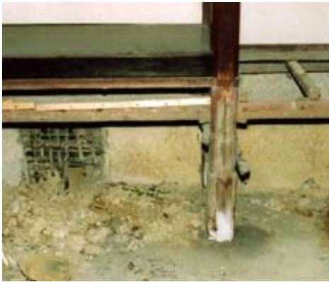
Photo 8: The base of the pillar in the sitting room(Photo was taken during the earthquake-proof renovation)
